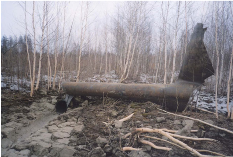
Fig. 1 Fracture of the gas-main pipeline in Yakutia at low climatic temperature
