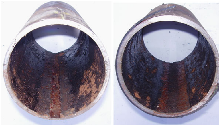
Fig. 6 Comparison of internal corrosion in two locations of the pipeline
